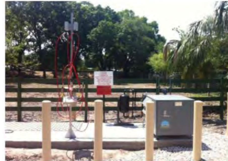
Compressor and Dual hose Time-fill post in Gulf Breeze, Florida
